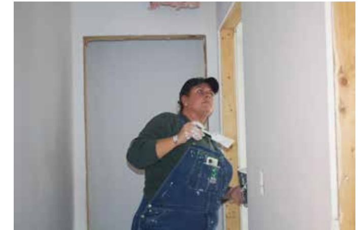
Maria Hynson uses a paint brush to paint the sides and corners of the walls that the paint rollers could not reach
